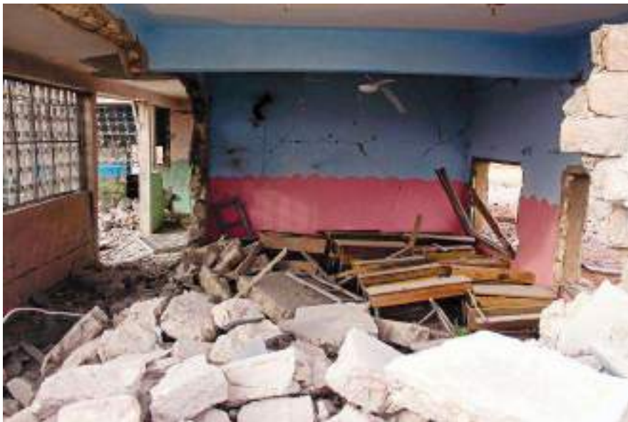
PHOTO: Russian airstrikes blasted through the concrete walls of a school in Atarib, destroying much of it. (SIJ)
