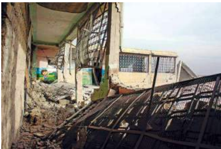
PHOTO: Russian airstrikes blasted open this school in Atarib, exposing the main corridor that led from the entrance to the classrooms. (SIJ)
